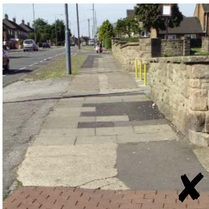
Farnborough Road - inconsistent paving
