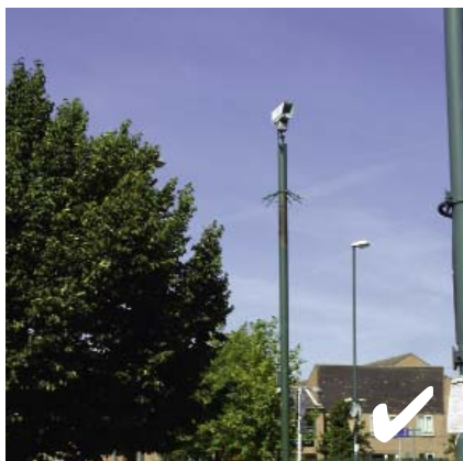
Arkwright Street/Radcliffe Street - CCTV equipment
