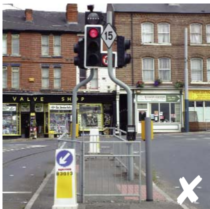
Radford Road/Wilkinson Street - cranked signal poles
