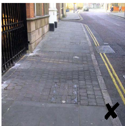
Goldsmith Street/Burton Street - no inset tactiles
