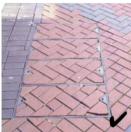
Pilkington Street, Bulwell - inset cover
