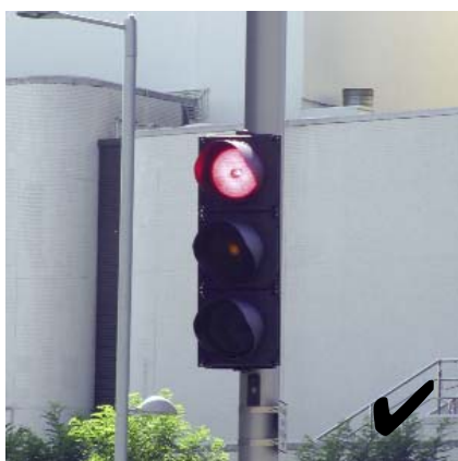
Burton Street/Talbot Street - Signal head without backing board
