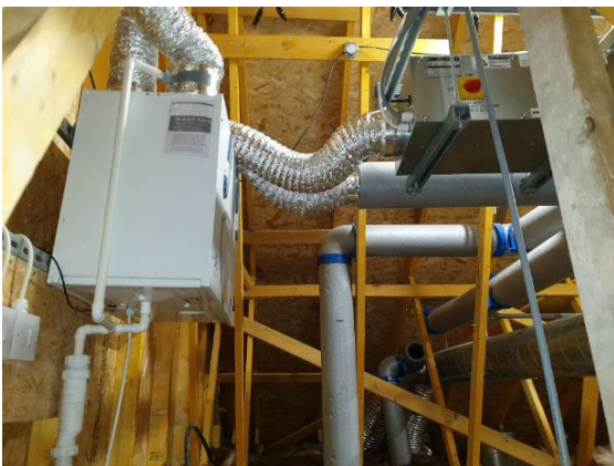
Figure 17: Example of MVHR and heater unit in cold loft with sections of uninsulated ductwork
